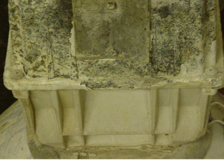
Example of improper material selection for lighting component in a food manufacturing plant.
