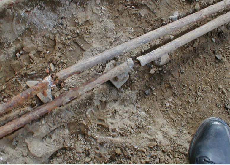
Corrosion found on conduit placed underground at a gas station.
