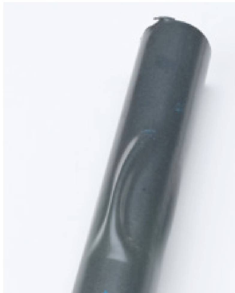
The PVC coating has blistered due to poor surface preparation of the galvanized zinc.
